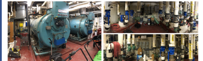
The High School Heating Plant is 38 Years Old – At Least 13 Years Beyond Its Life Expectancy
